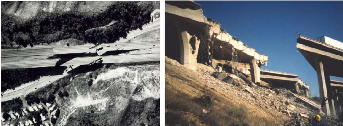
Figure 1. Gavin Canyon under crossing collapse in the 1994 Northridge earthquake
