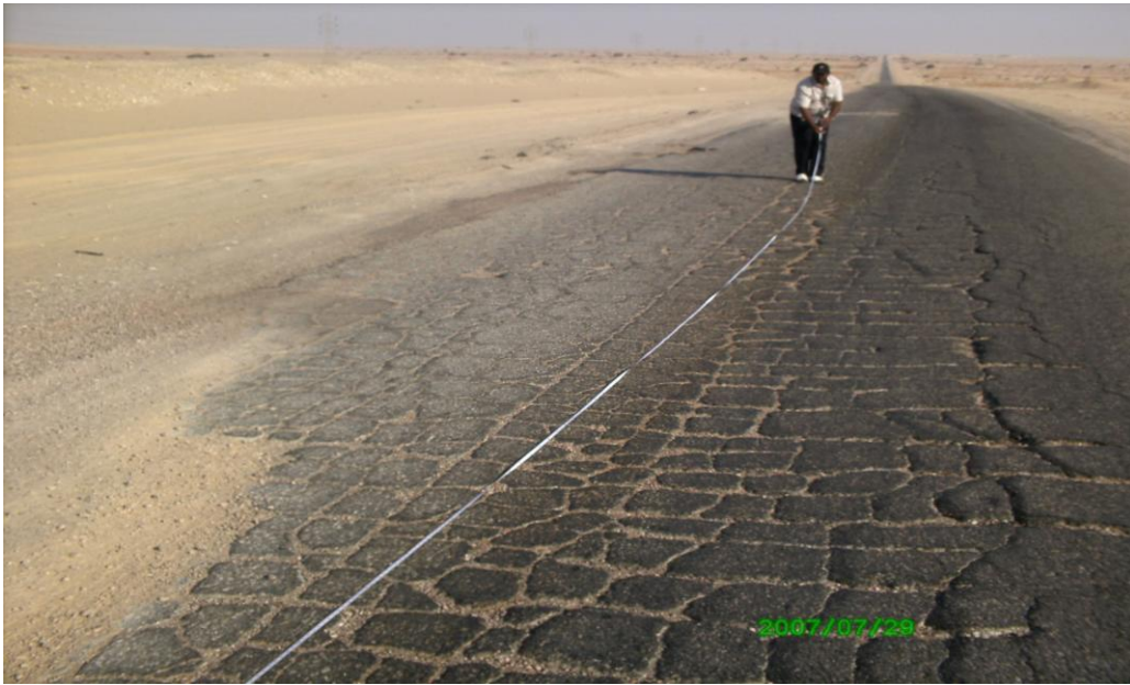
Figure (4): Identifying density of each distress and measure its severity
