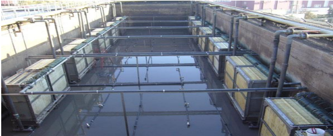
Figure 4: Shows Nitrogen Removal Plant in Romania.
