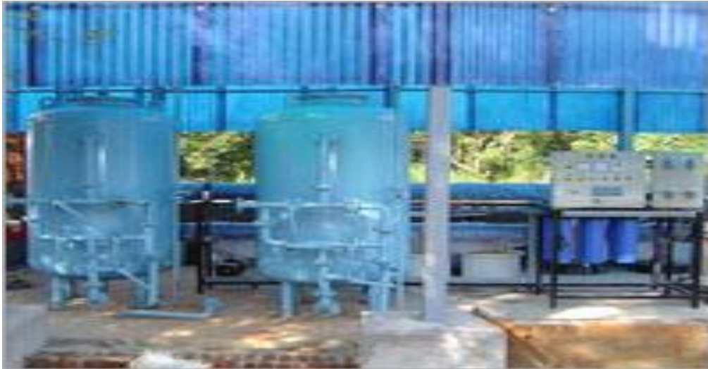
Figure 2: Shows a Tertiary Treatment Plant in Maharashtra, Indonesia.
