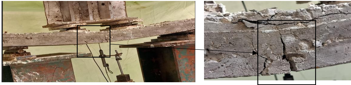
Figure 8. R.C. Failure Modes
